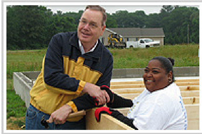
USDA Rural Development Under Secretary Dallas Tonsager helps Linda Diaz build her home at MHDC's Manchester Manor in Laurel, Delaware.
